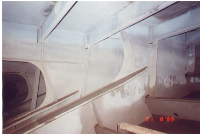
Figure 51: Ballast tank after 16 years.
