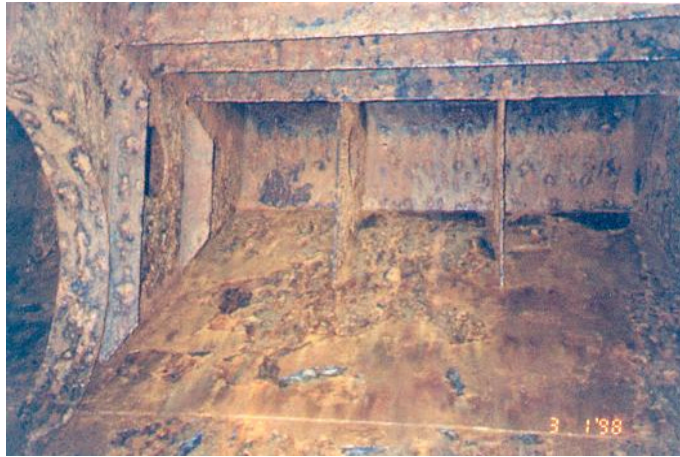
Figure 49: Coating condition after 13 years – Poor application.
