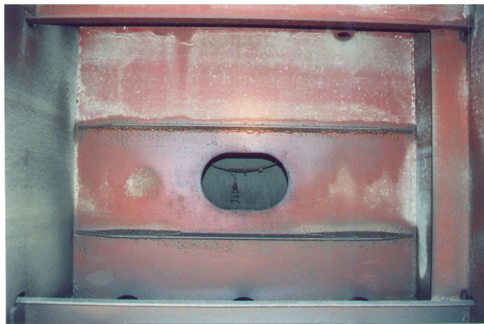
Figure 48: Coating condition after 13 years – Correct application.
