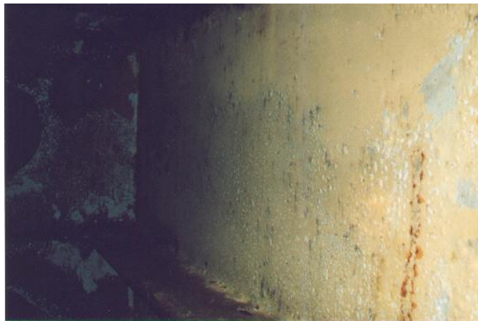
Figure 50: Ballast tank after 28 years.
