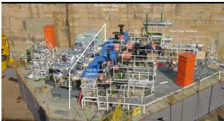
Figure 4.2: Typical compressor room
